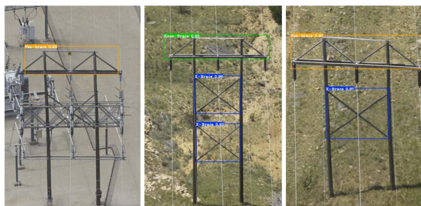
Fig. 16. Examples for brace type classification. Yellow boxes: V brace; green box: knee brace; and blue boxes: X brace.
